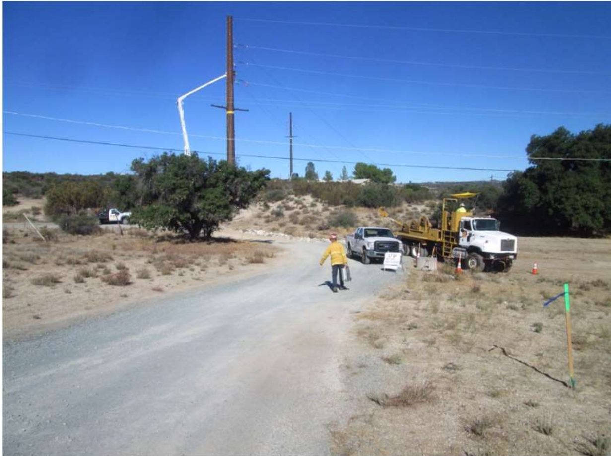
Photo 6: During preparation for wire stringing at the Z44294 stringing site (TL 6931), a fire patrol was observed inspecting the site in accordance with the CFPPP (MM FF-1).
