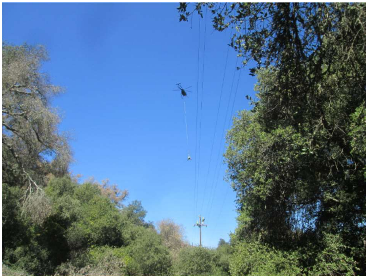
Photo 3: Along TL 682, longlines were utilized for equipment transport to pole sites and crews were observed scouting tree clearances from pole tops and relaying monitoring needs to staff below (Pole Z118148, above).
