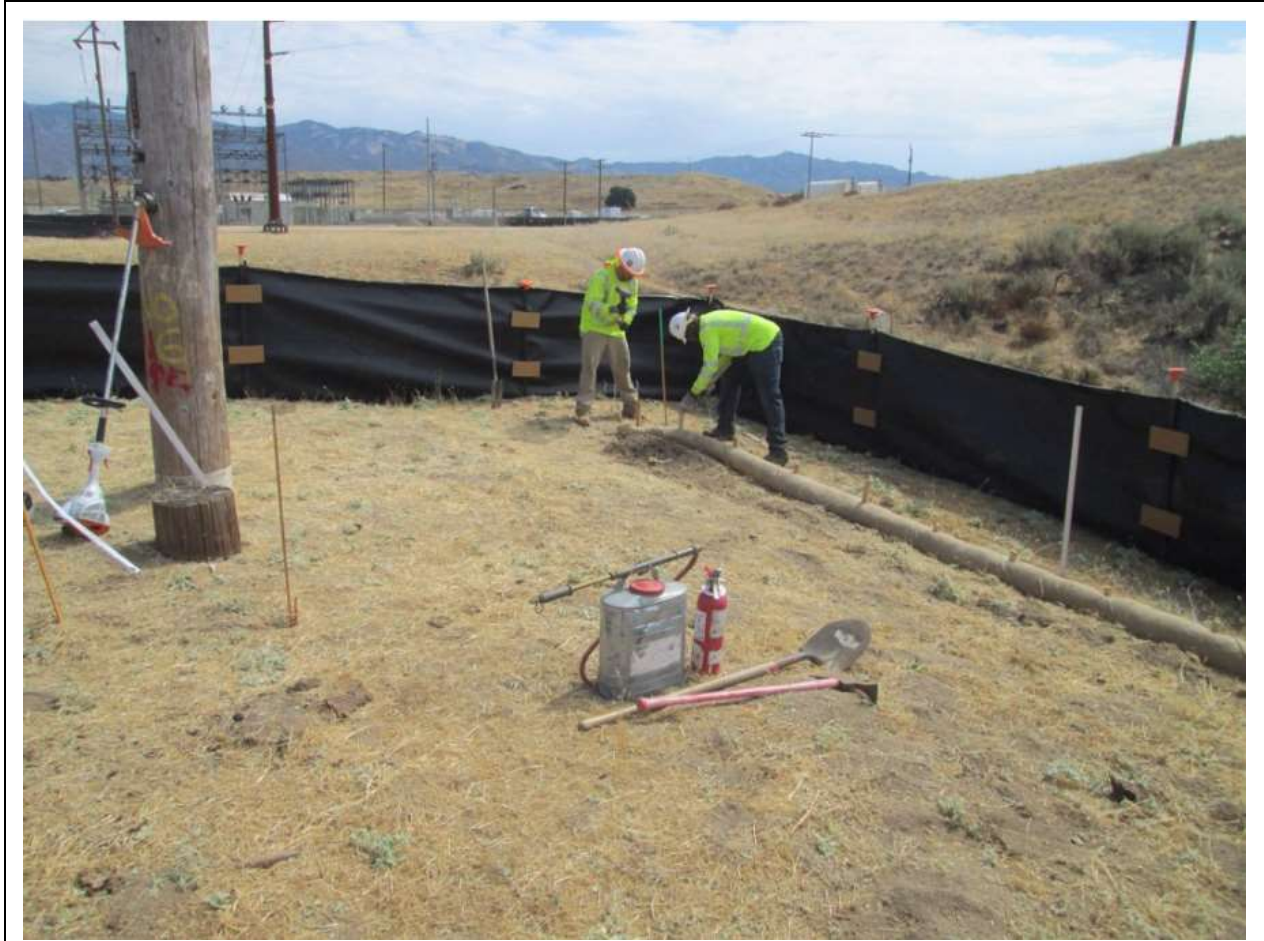
Photo 1: A crew observed installing fiber rolls (sediment control BMP) at Z210619 in accordance with the SWPPP, MM HYD-1, APM HYD-09, and MM BIO-7. The crew worked within the Stephens' kangaroo rat exclusion fence in accordance with MM BIO-31. Fire tools were observed on site in accordance with the CFPPP (MM FF-1).
