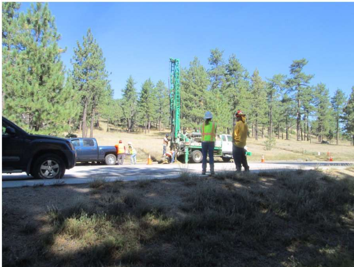
Photo 5: During geotechnical boring at B14 (C440), a biological monitor was observed on-site in accordance with MM BIO-3 and MM BIO-22, and a fire patrol was present in accordance with the CFPPP (MM FF-1).
