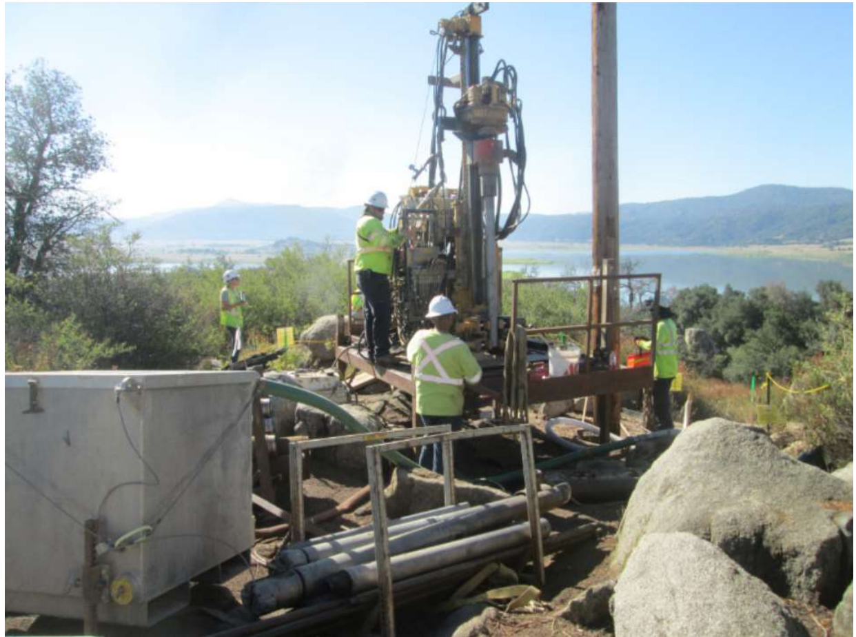
Photo 2: A construction crew was observed conducting micropile activities at Pole Z118168 (TL 682).
